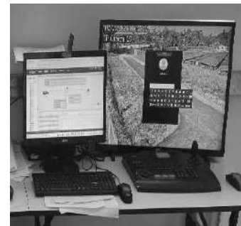
Remote security monitoring system
