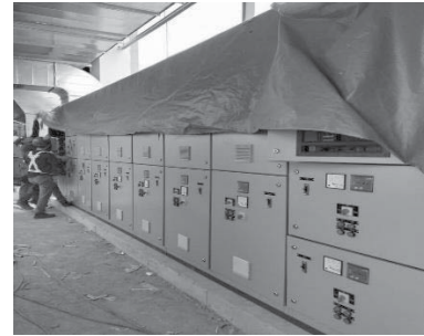
Motor control centre panels
