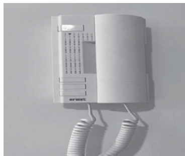
In-building telephone system
