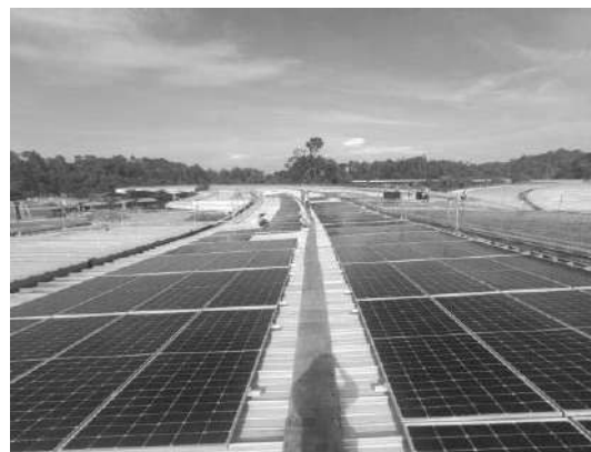
Overview of a rooftop solar PV installation
