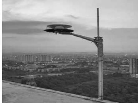
Lightning rod protection system
