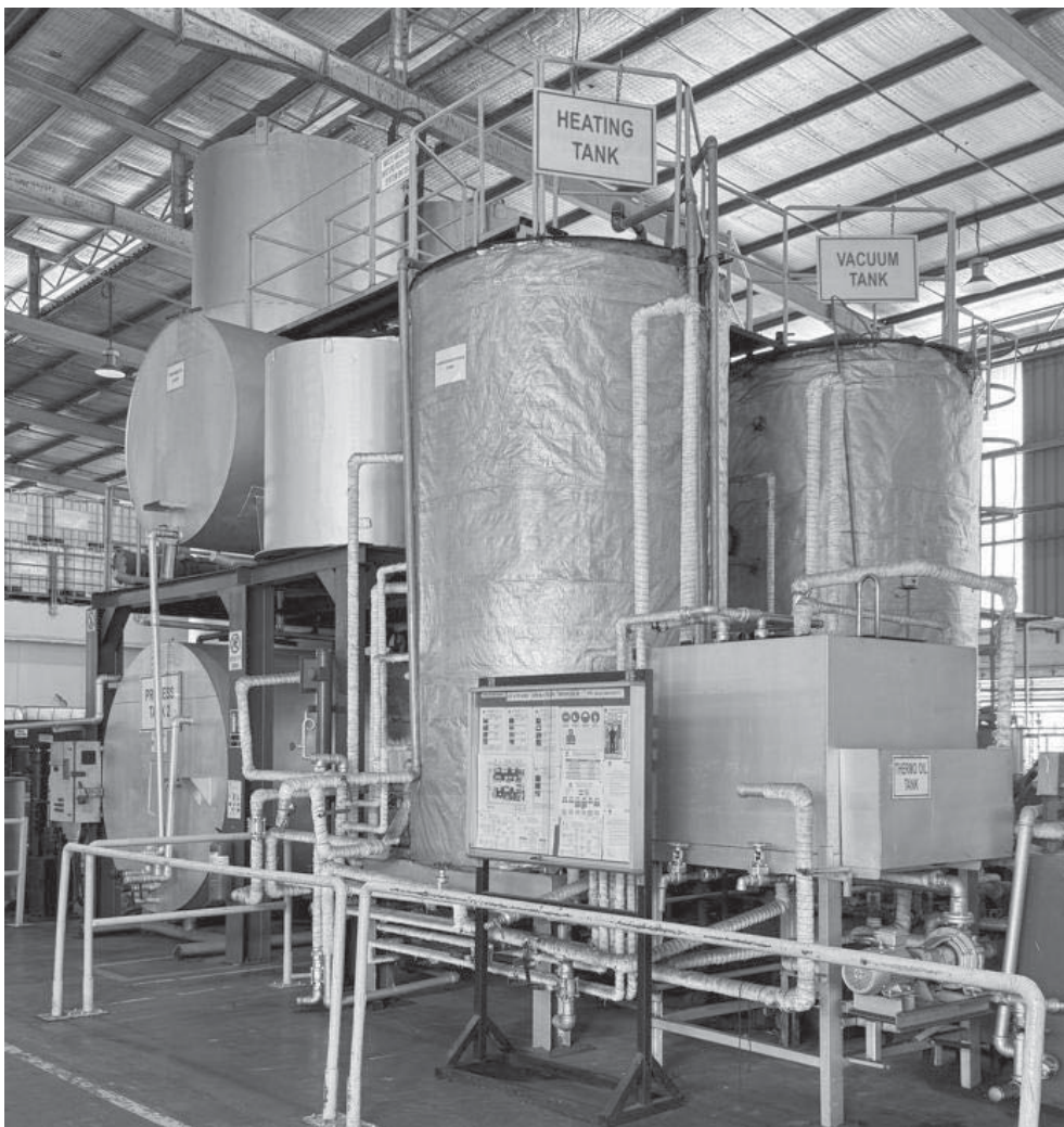
One of our waste oil recycling systems
