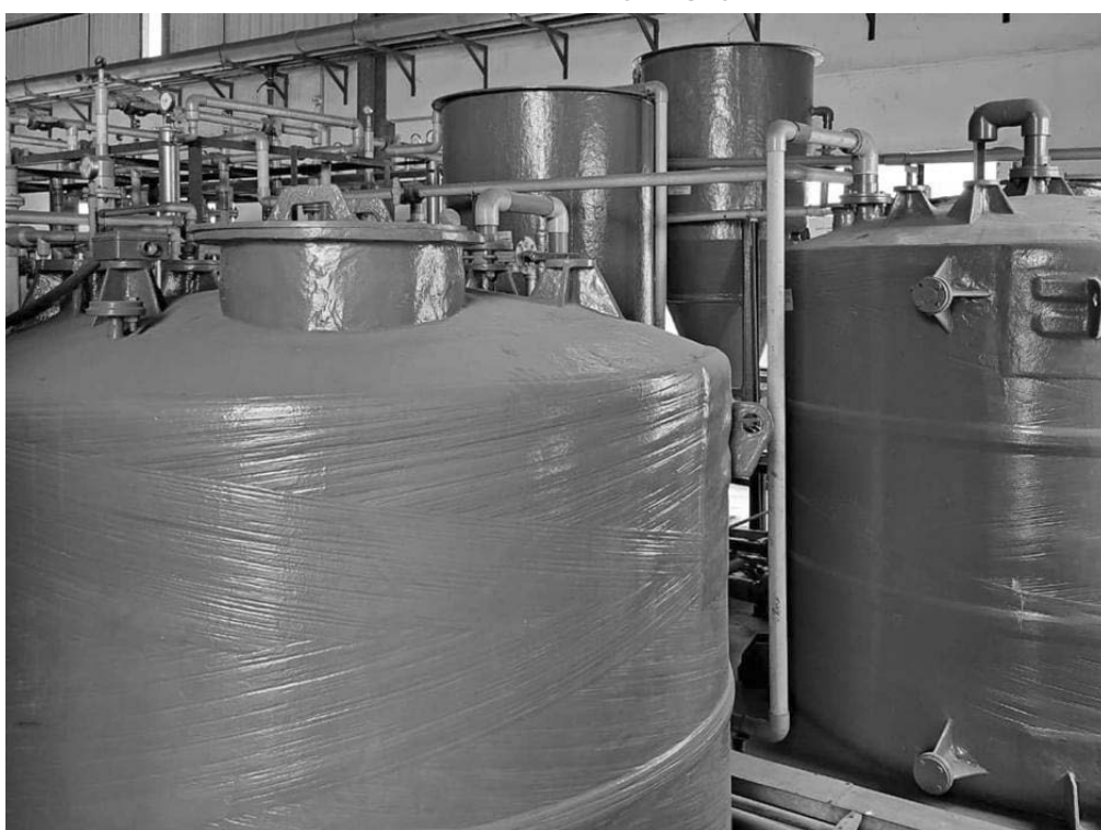
One of our waste acid recycling systems
