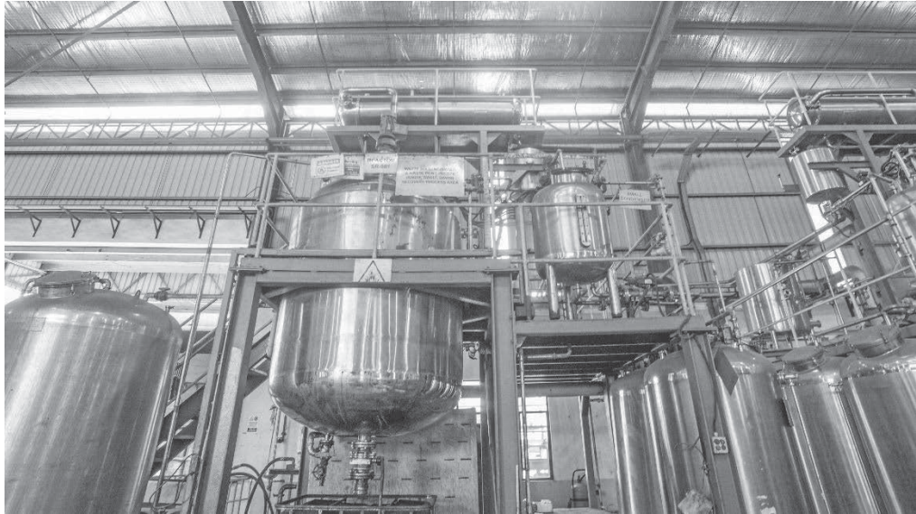
One of our solvent recycling systems
